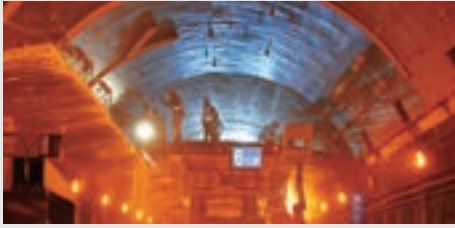
④ Central part of the ceiling panel cut off longitudinally
