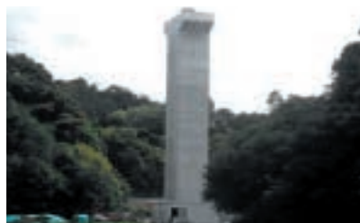
② Construction of the substructure for National Road Detour Bridge No. 1 at Naruse Dam
