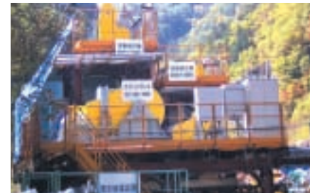
⑥ Dewatering facilities (horizontal screw press machine: \phi 1,000\text{mm} / \phi 500\text{mm} )
