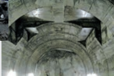
① Filling in a complicated cross-section (mounting area of emergency door in an evacuation connecting tunnel)
