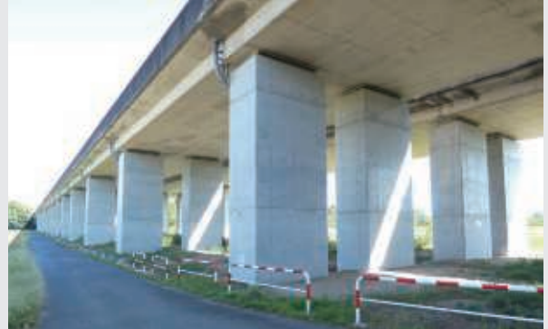
Horinouchi Daini Bridge and other 4 bridges anti-seismic reinforcement work on the Ise Expressway
